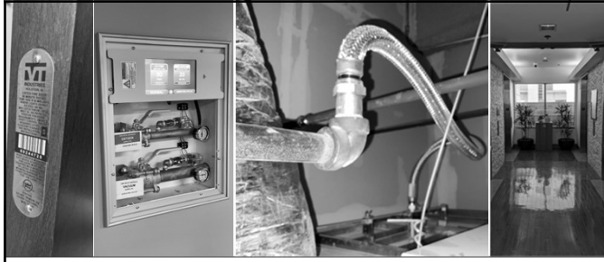
System Checklists HOW TO GUIDE FOR HOSPITAL PROJECT MANAGERS, DESIGNERS, AND CONTRACTORS
